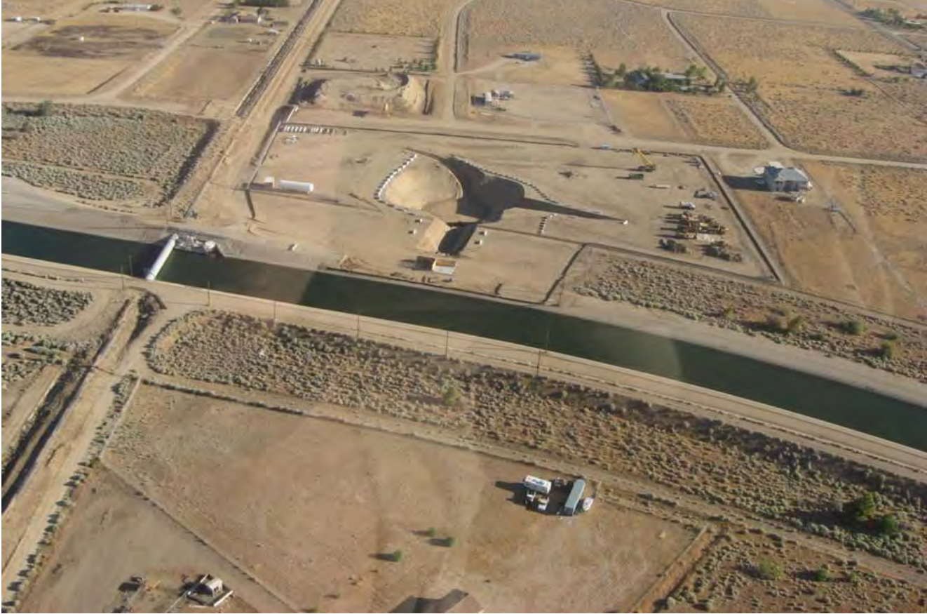
Neenach Temporary Pumping Station, construction site, looking northerly, taken September 16, 2010, by Aqueduct Aerial Patrol.
